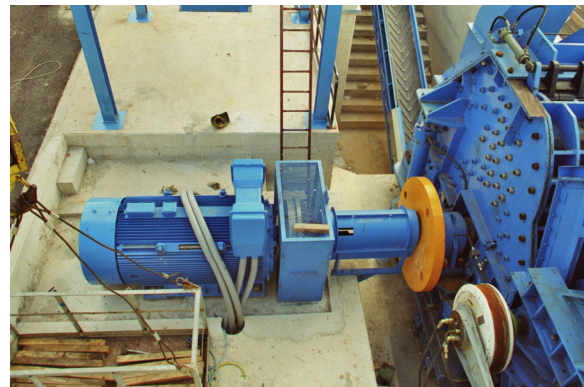
Pic. 5: Shredder drive with hydraulic coupling
